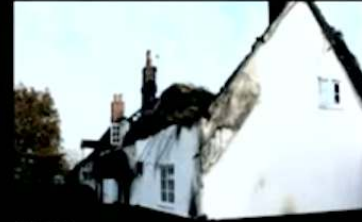
Amount of damage done by fire
