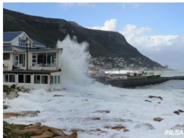
Waves smash against the windows of Kalk Bay harbour restaurants. The large picture windows of both Harbour House and Live Bait were smashed in, resulting in serious damage to the interiors and one minor injury. Photo: Leon Lestrade.
